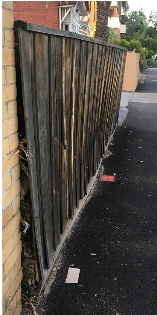
Figure 3. Practical issues of ambiguity as to the limits of boundary occupation. At the few cm level, this fence exhibits: (a) an offset from an abutting boundary on the same alignment; (b) non-verticality; (c) lack of horizontal straightness; and (d) a somewhat rough and ambiguous surface. (Melbourne, Victoria)
